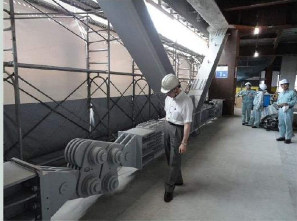
2250 kN damper installed in the building
