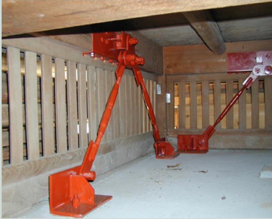
Dampers installed in the space under the floorboards
